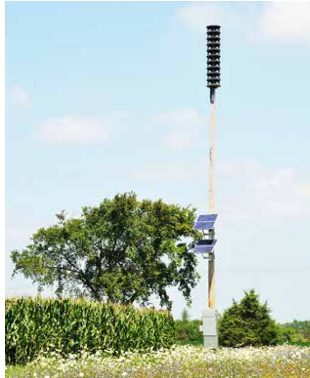
Installation of early warning systems to contribute to public safety and increase preparedness for future storms.
