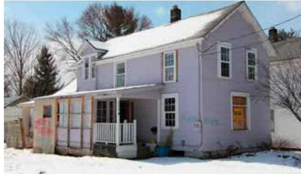
Example of flood damage to a home in the Owego Flats neighborhood.
