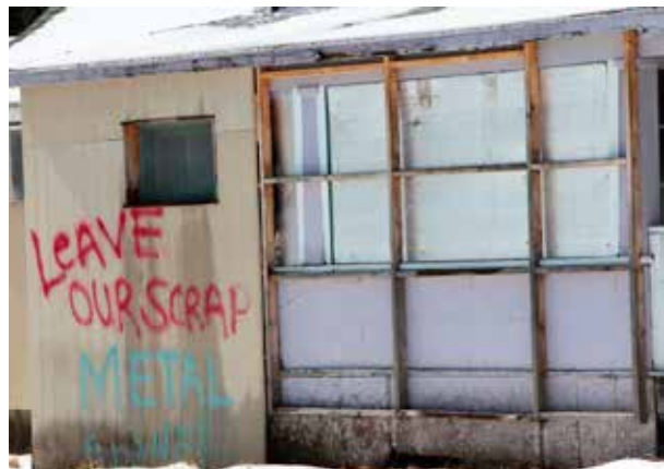
Low-lying neighborhoods in Owego suffered extensive damage.
