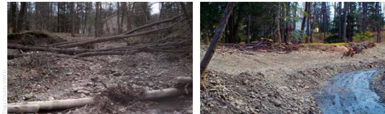
Town of Owego Emergency Stream Intervention (ESI) site before and after images.
